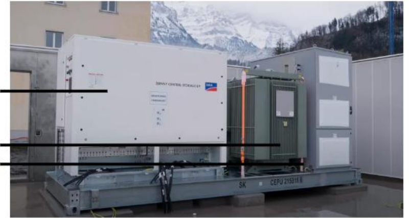
Transformator Oil Containment
